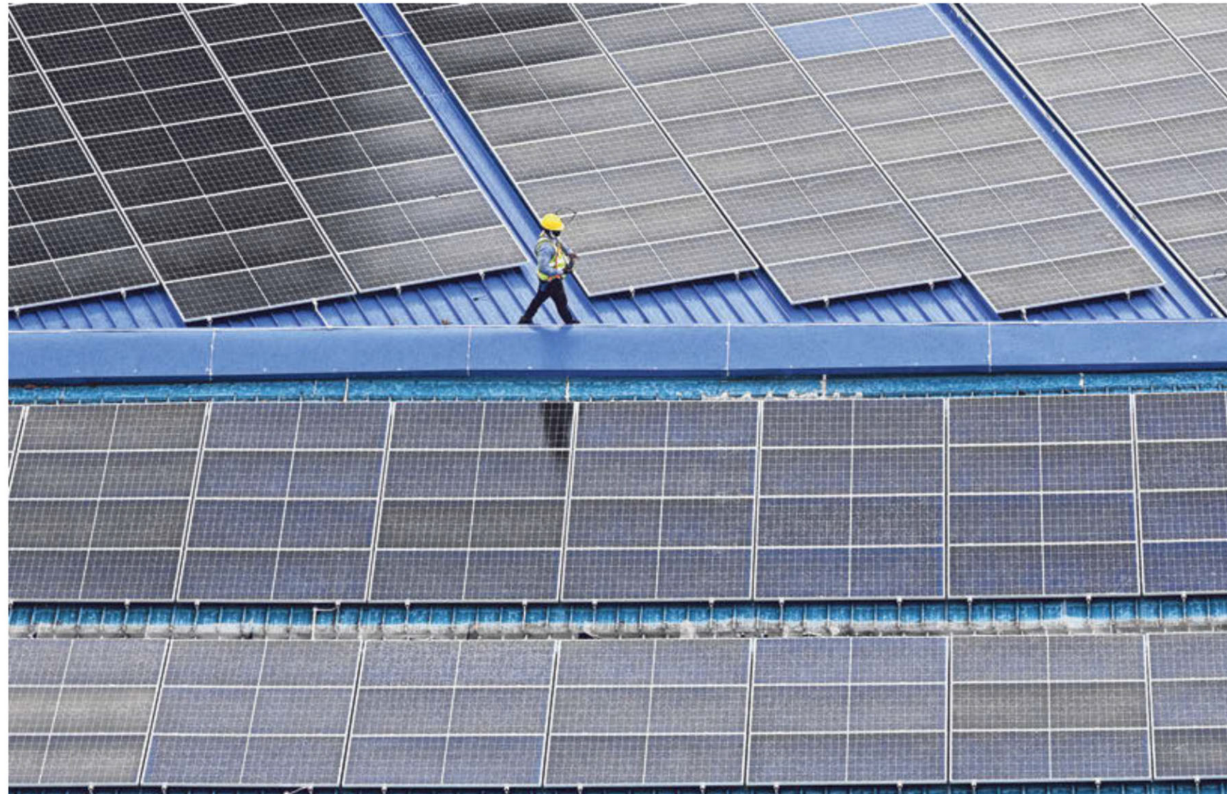
A worker installing rooftop solar photovoltaic panels at Shell Havelock Service Station last month. Besides tapping solar energy, Singapore has also identified nuclear energy as having the potential to supply about 10 per cent of the country's energy needs by the middle of the century. ST PHOTO: LIM YAOHUI
