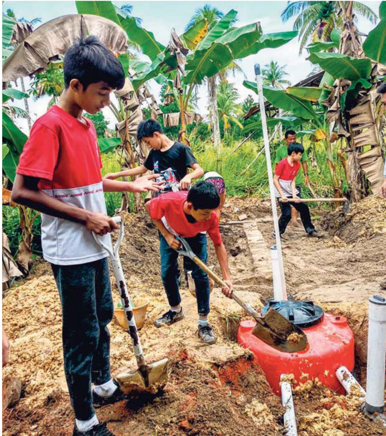
Students from Juying Secondary School helping to build a Safe Water Garden water sanitation system in Bintan in 2018, before the Covid-19 pandemic. Now, all sessions are conducted online due to travel restrictions, and the sanitation systems are constructed by staff from LooLa, an eco-adventure resort in Bintan. PHOTO: SAFE WATER GARDENS/ LOOLA
