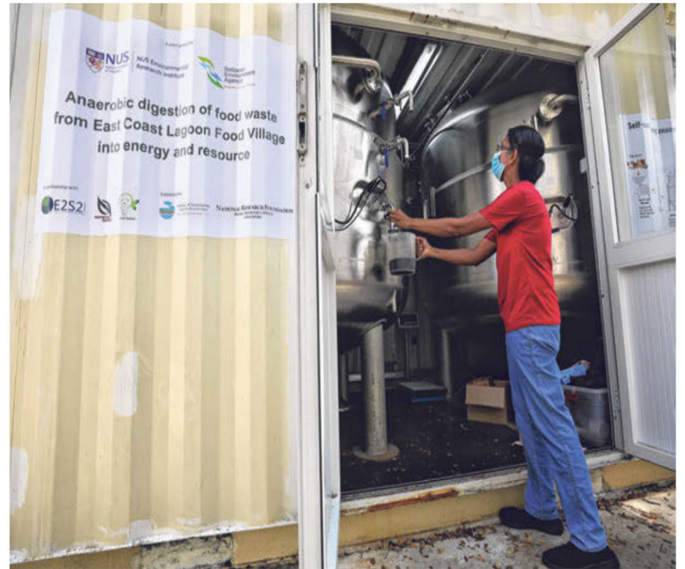
2 The operations associate retrieves a sample – to be tested for methane levels – from the anaerobic digester in the self-sustaining anaerobic digestion system that converts the food waste to biogas and fertiliser.
