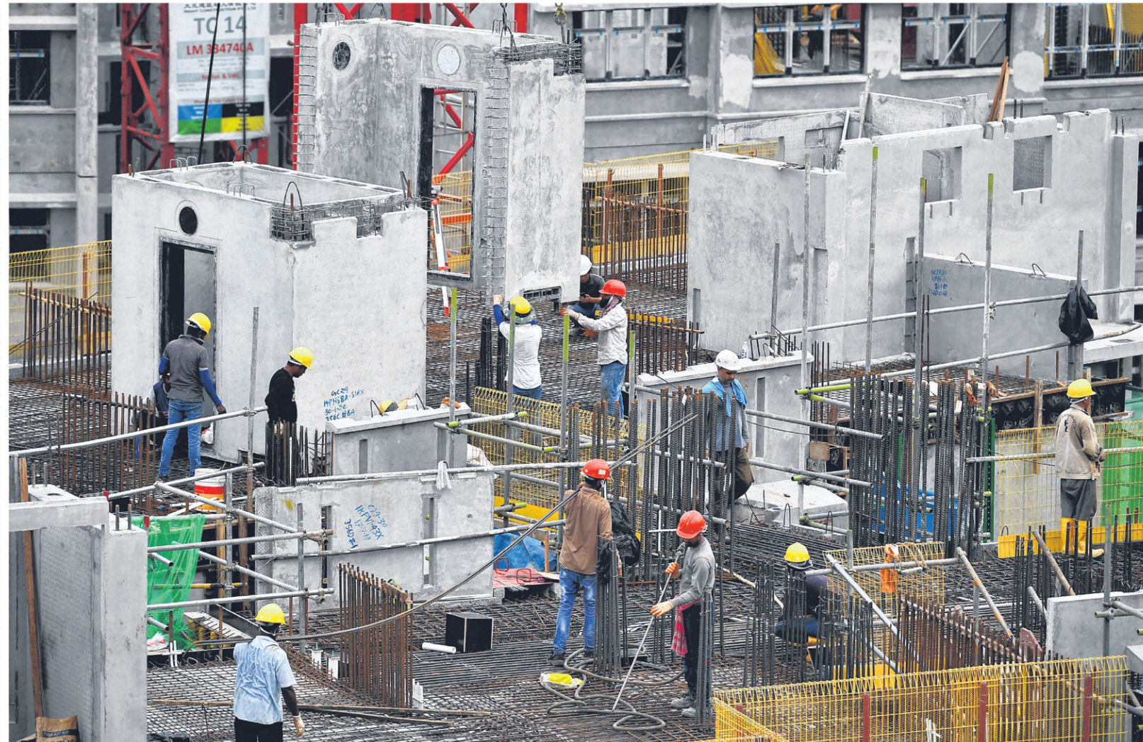
Workers at the construction site for HDB's Ubi Grove project. Covid-19 has made clear that a fundamental review is needed of the desired outcomes of economic and other activities as well as full costing of foreign labour. These will bring the numbers of foreign workers into proper balance, say the writers. ST PHOTO: LIM YAOHUI
