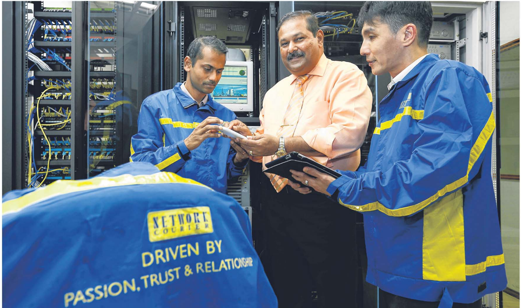
Mr V.S. Kumar (centre) with system administrator Tamil Selvan and operations supervisor Allen Koo in the Electronic Data Processing room, where high-end servers are stored and software such as the Virtual Client system is managed. The system can route job instructions directly to courier staff and has time-entry devices such as biometric finger and vascular scanners. BT FILE PHOTO
