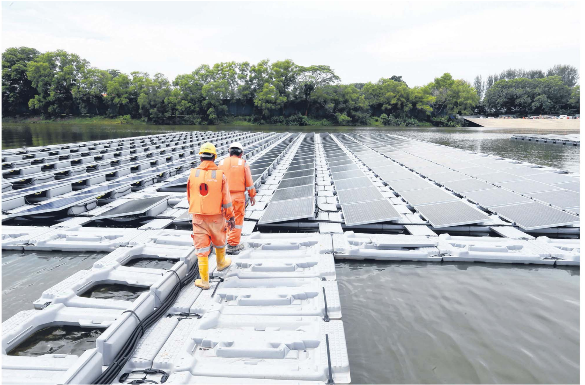
The floating solar photovoltaic cell test bed is an amalgam of 10 different systems. Each system, consisting of solar cells that can convert sunlight directly into energy, has a peak capacity of 100 kilowatts, enough to power 30 four-room HDB flats for a year. More than 150 sensors and other monitoring devices will capture the data to see which performs best. ST PHOTO: LAU FOOK KONG
