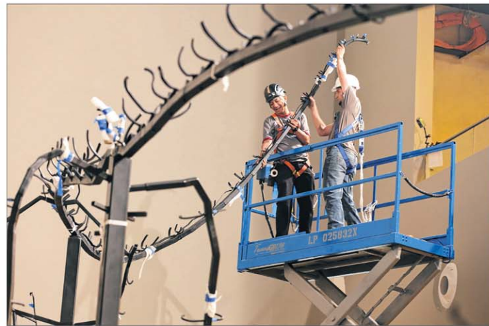
Workers installing a mount for one of the sauropod skeletons last August.
